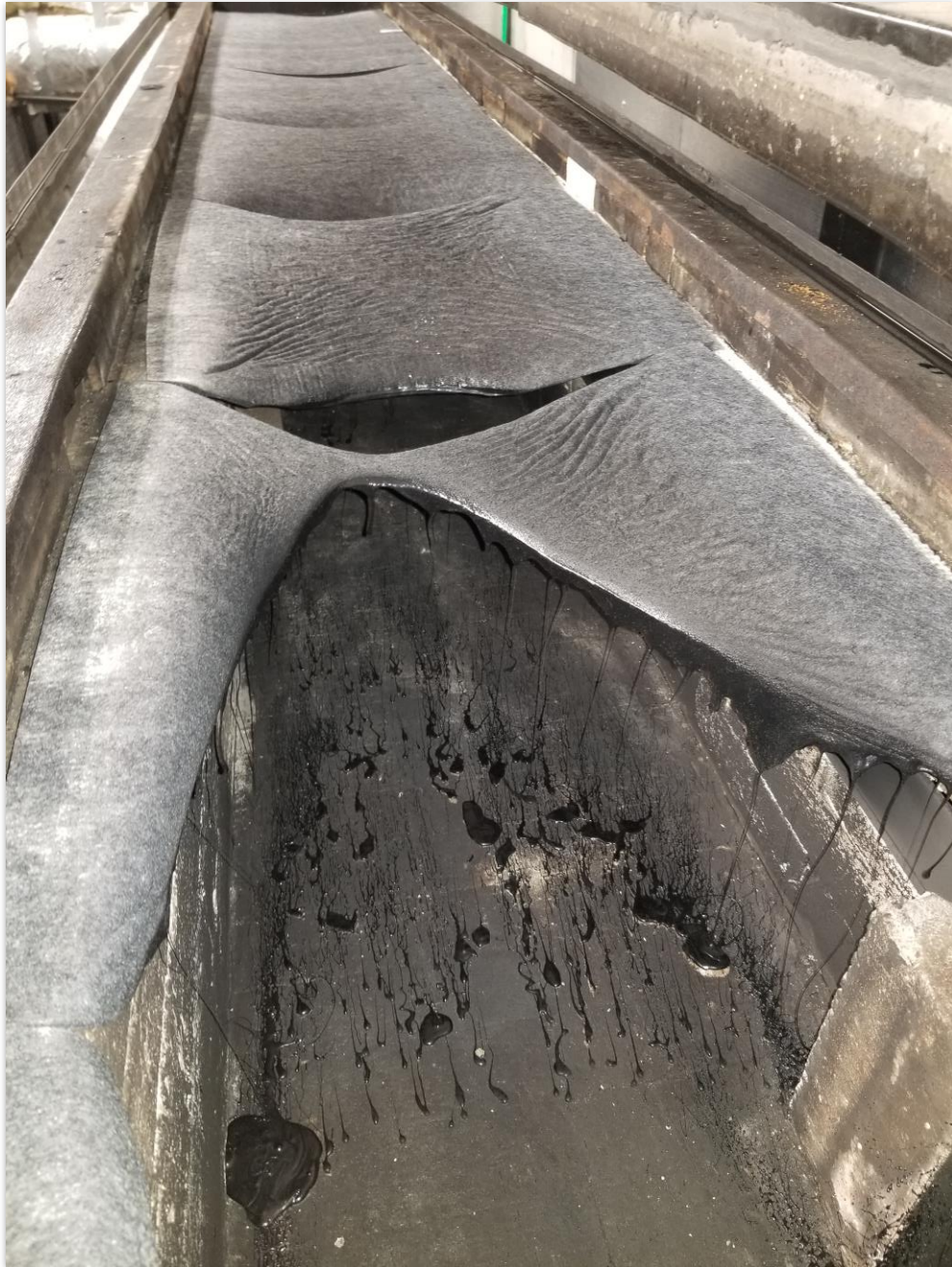
Figure 3 - Close-up of melted board
